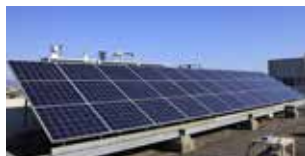
Solar panels of TUT
